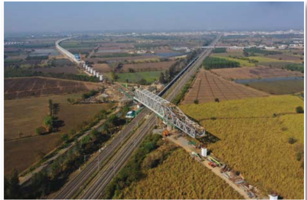
100 m long 'Make in India' Steel Bridge launched over four Railway Tracks in Surat, Gujarat
